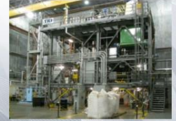
Full commercial scale tubular (fixed-bed) FT reactor at TRI's demonstration facility in Raleigh Durham, NC.
